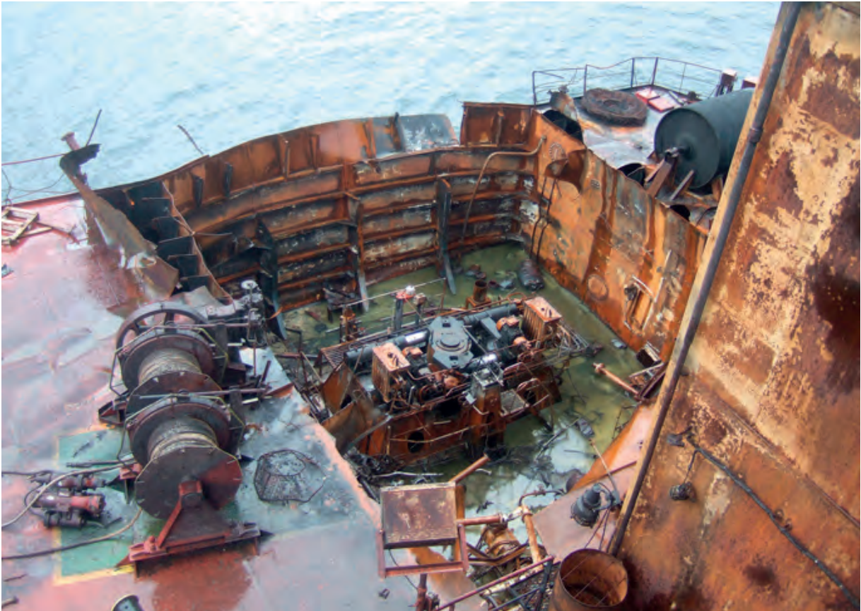
Figure 2: Exposed steering gear
