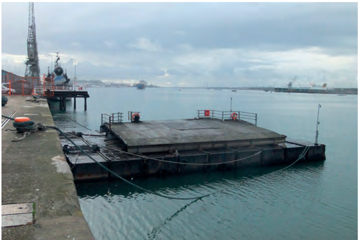
Figure 3: The linkspan with missing ramp
