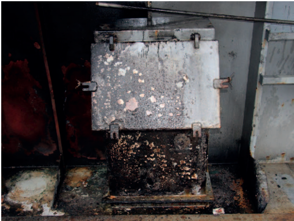
Figure 2: Hold ventilation cowl damage
