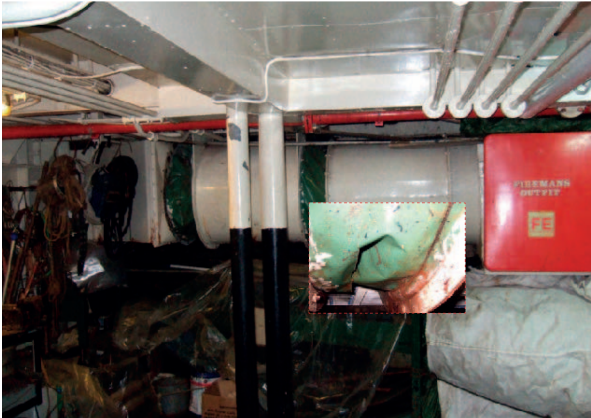
Figure 2: Forward store - vent trunking from cargo hold to deck vent
