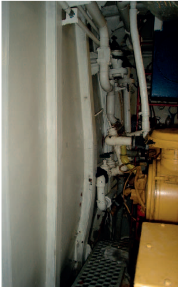
Figure 3: Bulkhead and frame damage
