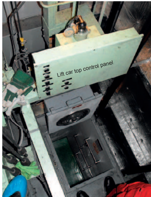
Figure 2: Escape hatch and lift car top control panel
