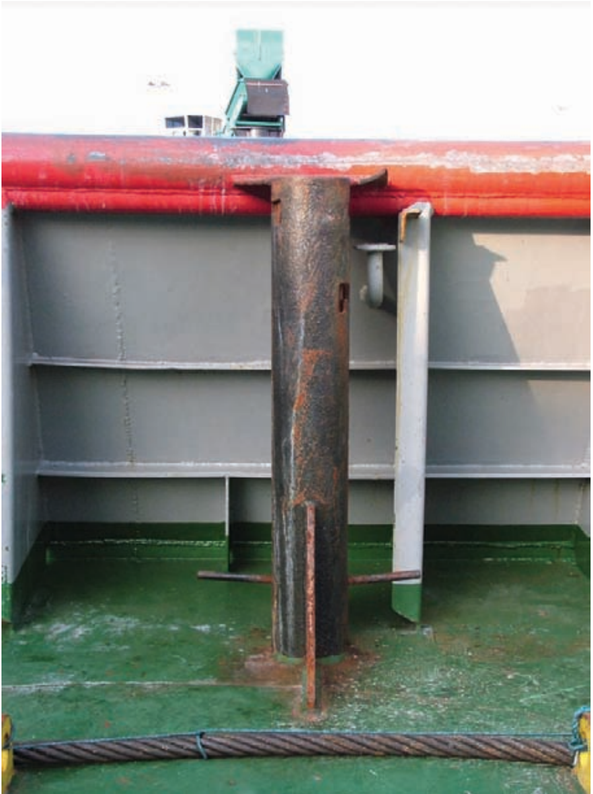
Figure 2: Damage to Norman Pin socket
