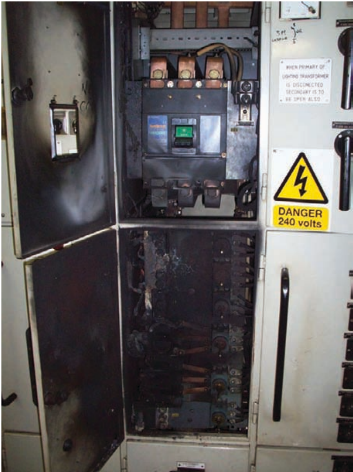
Damage to cable insulation and fittings
