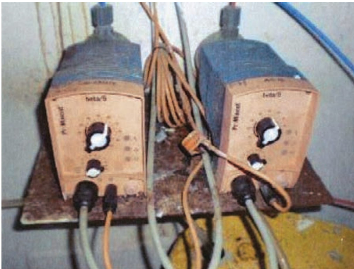
Figure 2: Pool dosing pumps
