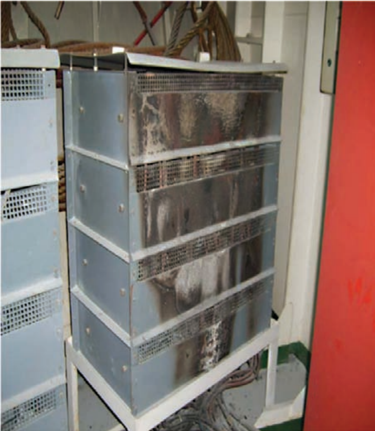
Figure 1: Bow thruster electrical resistor cabinet
