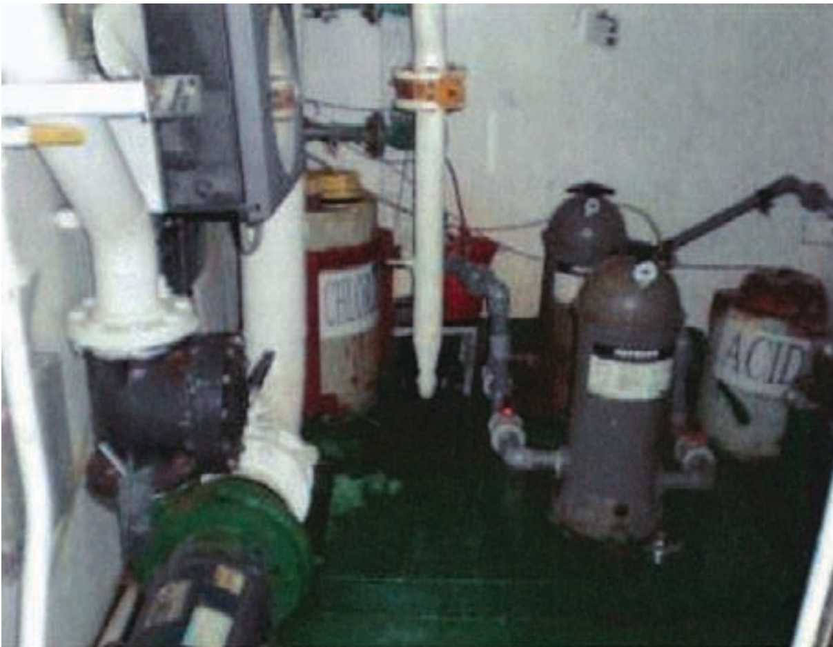
Figure 1: Pool machinery room
