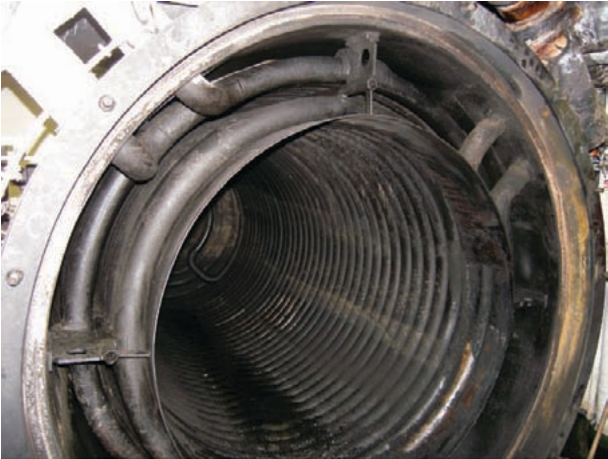
Thermal oil heater furnace
