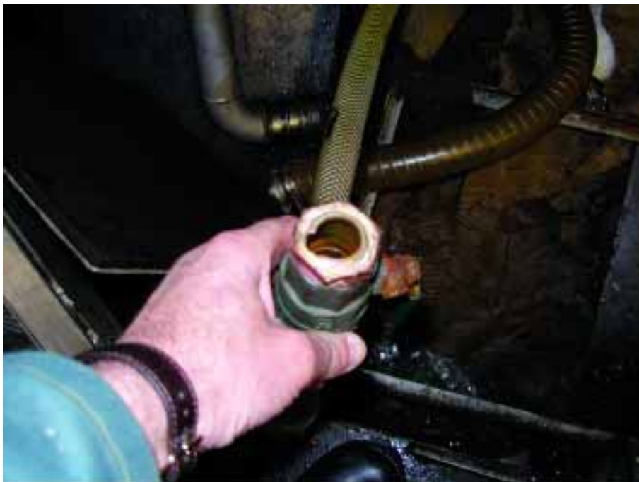
Sheared fitting after accident
