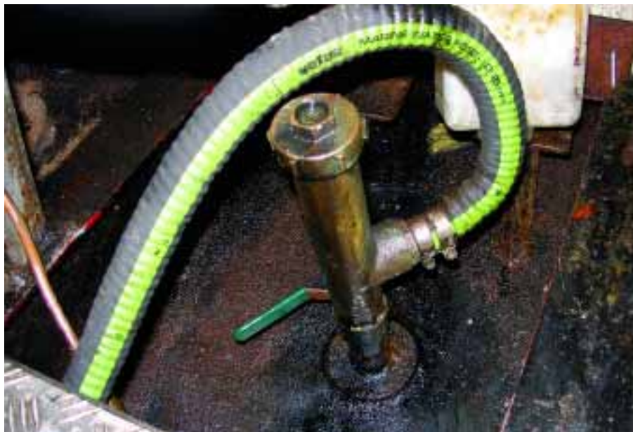
Similar sea water inlet before accident
