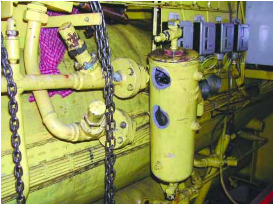
Figure 2: Damage to the inlet and outlet pipes
