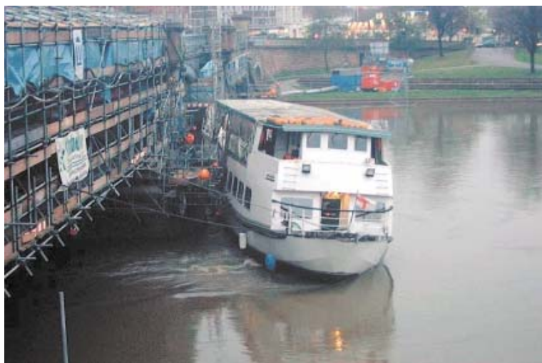
Figure 1 Vessel pinned to bridge (note: flow of river water by bow)
