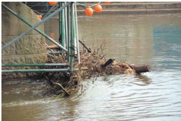
Figure 2 'Flotsam' on southern buttress
