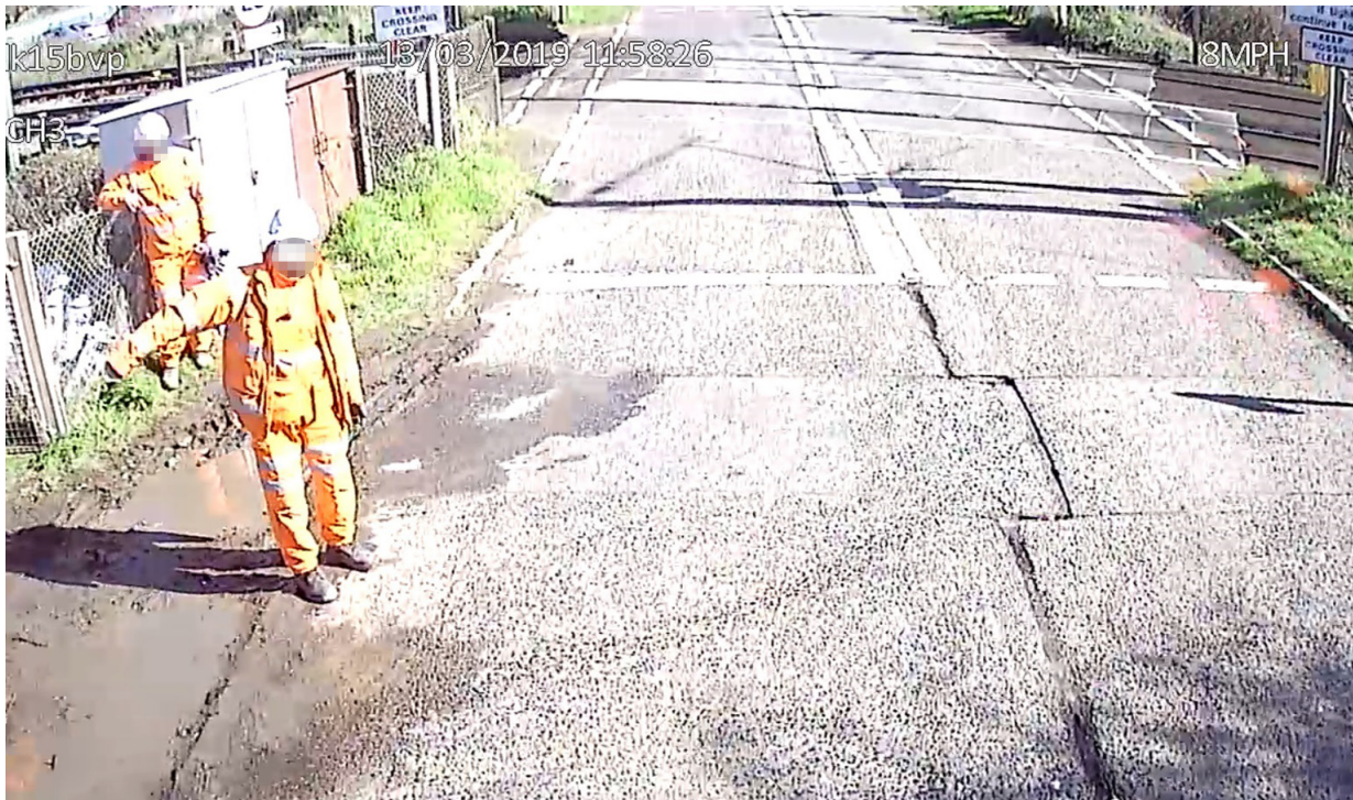
Figure 7: Lorry front camera view of banksman waving concrete delivery lorry forwards towards the level crossing (courtesy of Euromix Concrete)
