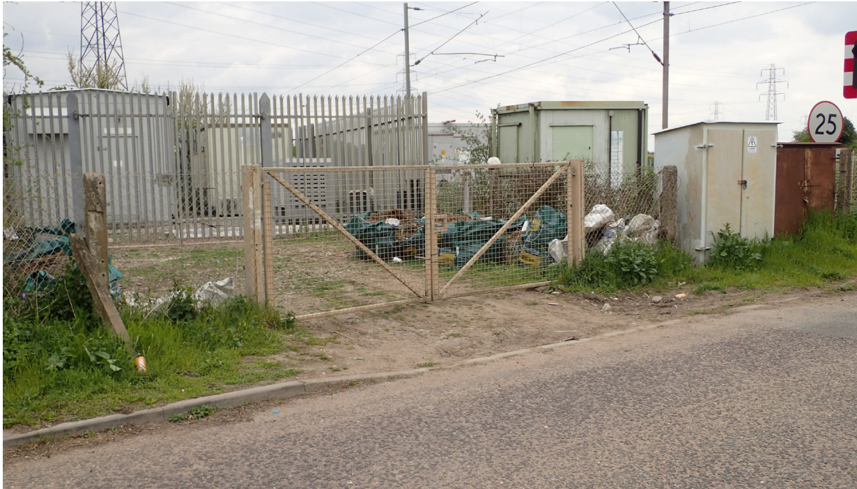
Figure 5: Mucking principal supply point compound
