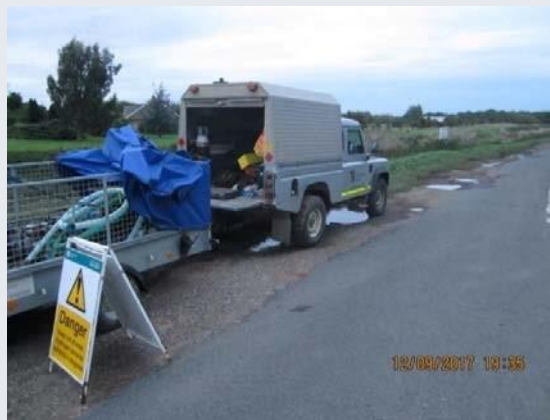
Fisheries hydrogen peroxide dosing equipment in action.
