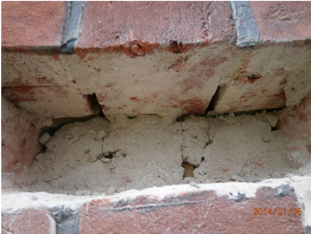
Figure 10: Example of missing mortar in perpend joints. Looking upwards at exposed bricks in the upper course at the top of the void, the extent of mortar in the perpend joints can be seen. In this example, the perpends can be estimated to be approximately 50% filled.
