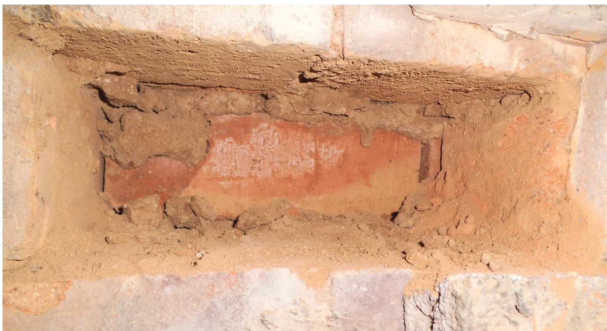
Figure 8: Exposed collar joint showing area of missing mortar. Some mortar remains attached (e.g. in the top left of the exposed inner leaf), with other regions showing staining (e.g. bottom right of the exposed inner leaf). The central portion of the inner leaf shows no staining, suggesting little or no mortar was present.
