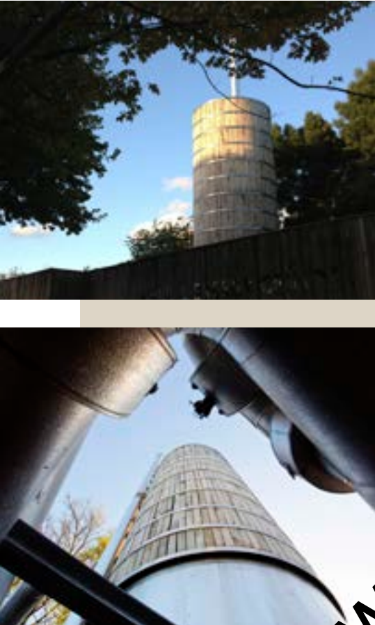
Bunhill Heat and Power, courtesy of Islington Council
