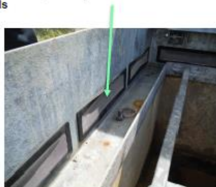
The reservoir over-spilled through air vents in the roof covers, causing the vents to distort outwards
