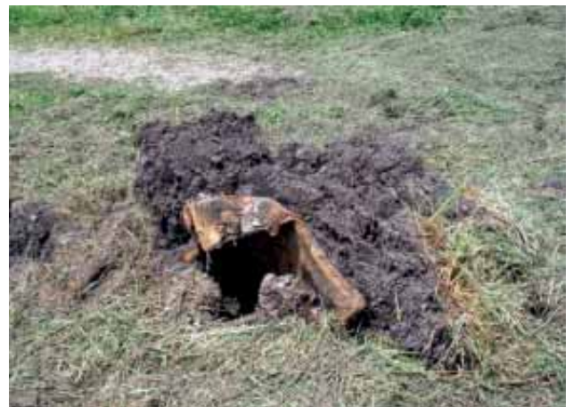
One of many items of debris encountered in the imported topsoil during remedial works
