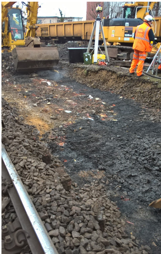
Figure 15: Excavation of the track bed close to the point of derailment on 14 January 2017 (photograph courtesy of Network Rail)
