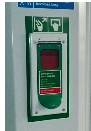
Release not pulled (normal position in service)
