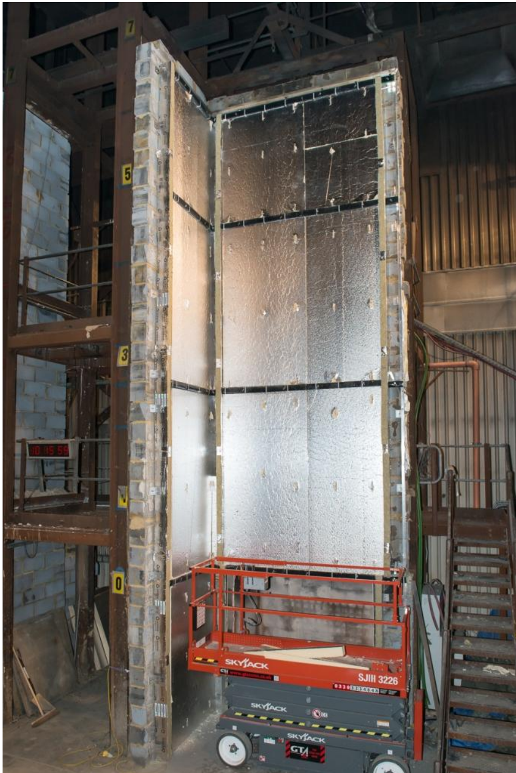
Figure 7. Installed cavity barriers. PIR insulation panels cut to fit and skewered onto 'L'-brackets.
