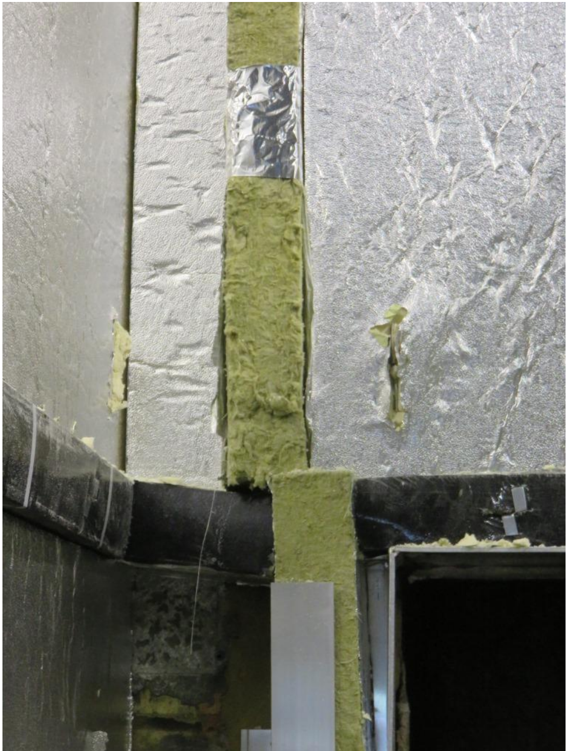
Figure 5. Vertical cavity barrier staggered at the height of the combustion chamber opening.
