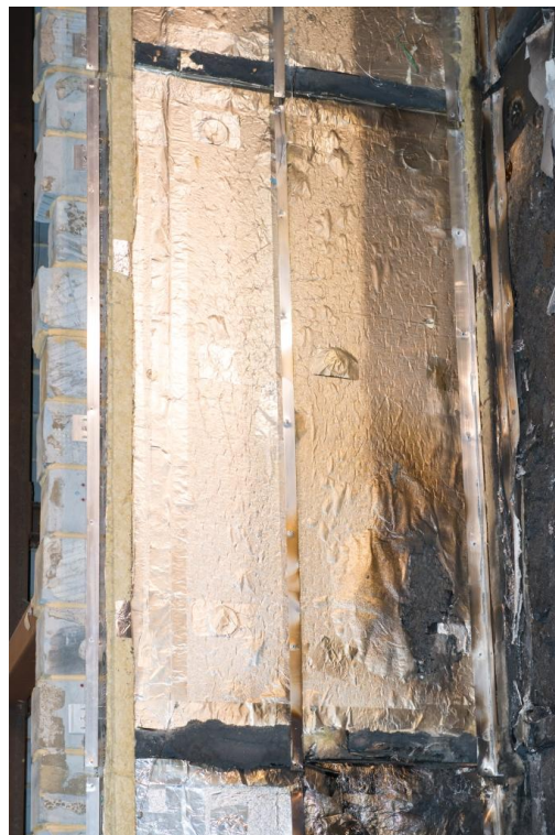
Figure 32. Damage to cladding system beneath ACM panels on wing wall between the second and third horizontal cavity barrier (approximately 2400-4700mm above the height of the combustion chamber).
