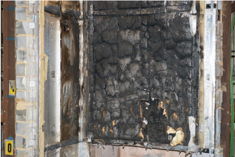
Figure 29. Damage to cladding system beneath ACM panels directly above the combustion chamber.
