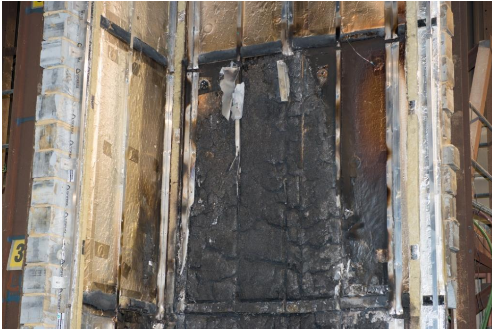
Figure 31. Damage to cladding system beneath ACM panels between the second and third horizontal cavity barrier (approximately 2400-4700mm above combustion chamber).
