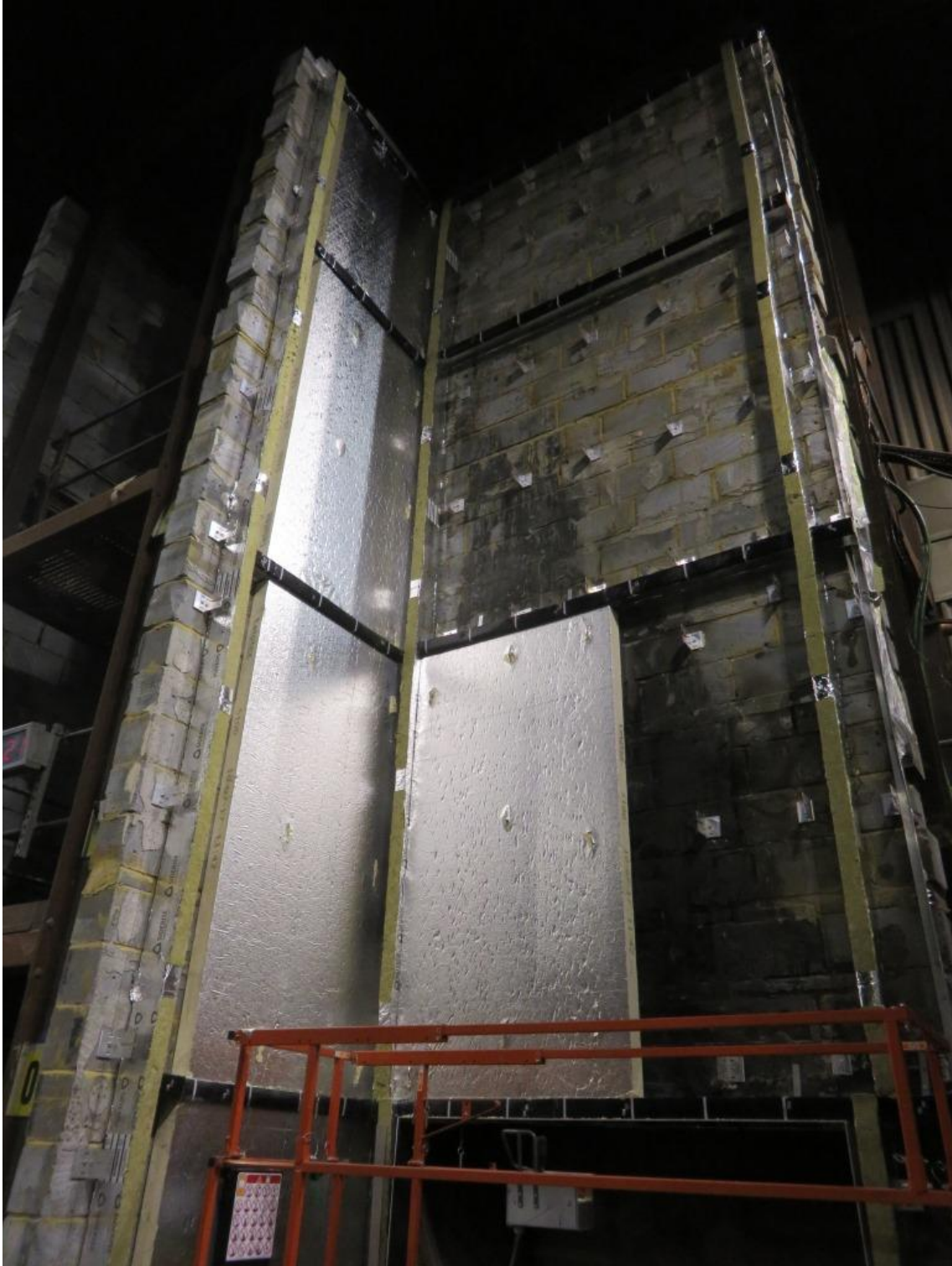
Figure 3. Location of 'L' brackets (partially visible), cavity barriers and PIR insulation panels.
