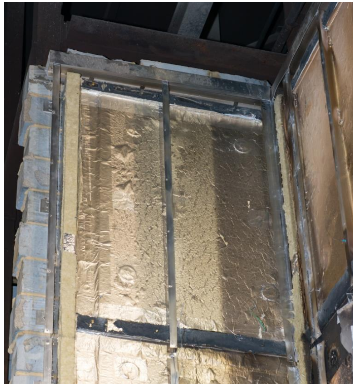
Figure 34. Damage to cladding system beneath ACM panels on wing wall between the third and fourth horizontal cavity barrier (approximately 4700-6360mm above the height of the combustion chamber).
