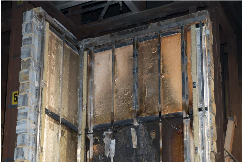
Figure 33. Damage to cladding system beneath ACM panels between the third and fourth horizontal cavity barrier (approximately 4700-6360mm above the combustion chamber).
