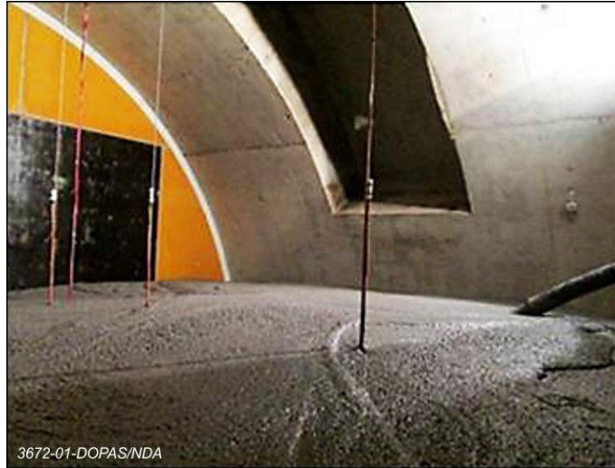
Figure 17 Casting of low pH concrete plug for the containment wall of the FSS Experiment
