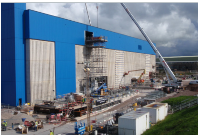
Rutherford provide insurance for buildings under construction, such as the now-completed EPS waste store at Sellafield
