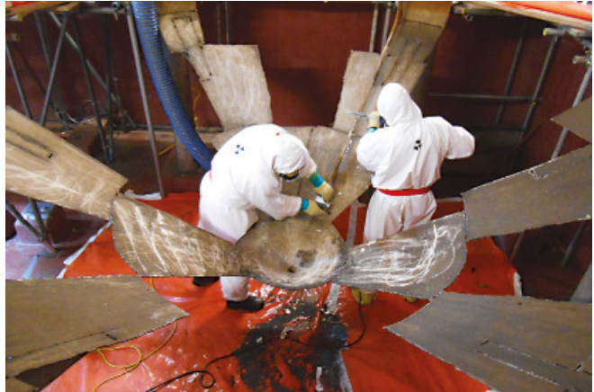
Cutting up the last delay monitoring tank at the Bradwell ponds in preparation for Care and Maintenance
