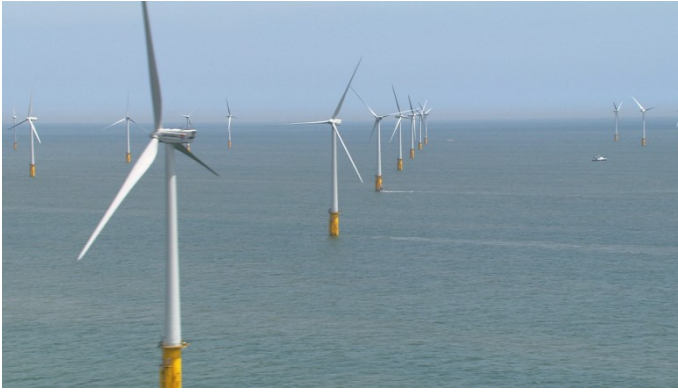
Thanet Wind Farm in Kent – the world's biggest offshore wind farm – will reduce the UK's need for imported energy (Photo: Vattenfall)
