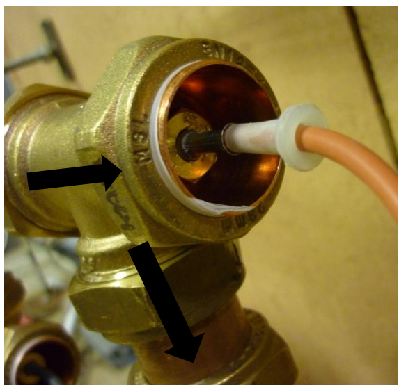
Figure 32: Adapted compression tee fitting to provide compression gland mounting of sensors
