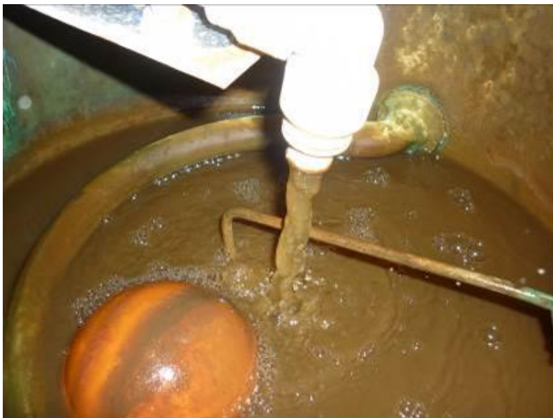
Figure 71: Test house installation – example of heating system water quality
