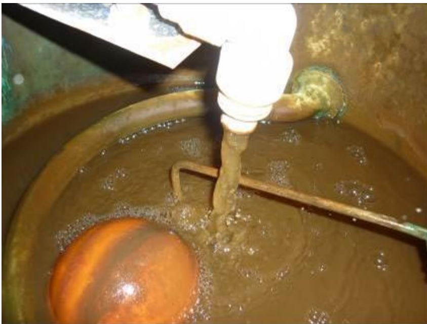
Figure 43: Test house installation - water quality
