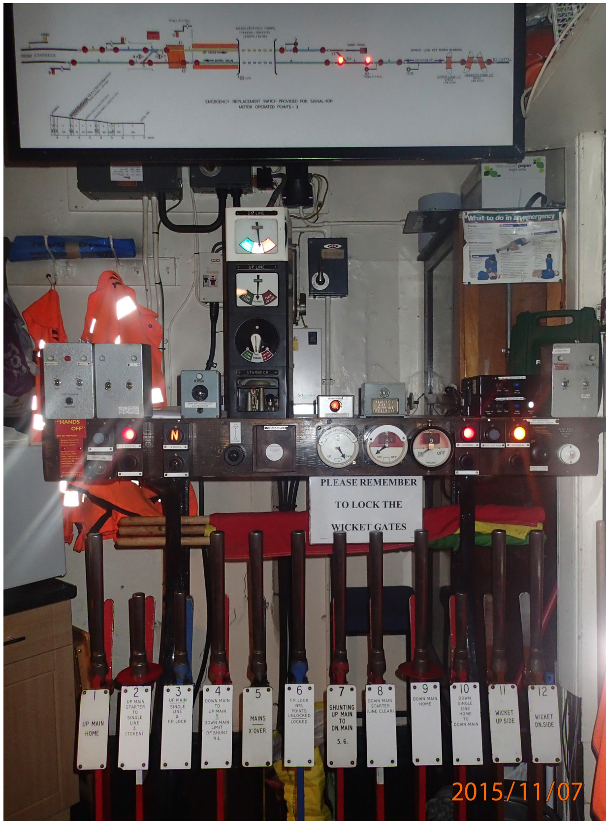
Figure 5: Knaresborough signal box lever frame
