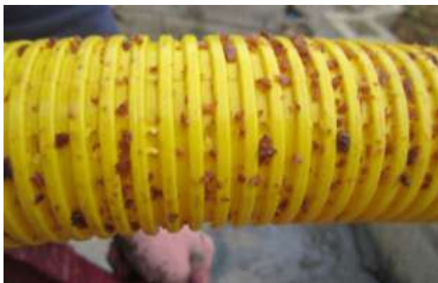
Figure 3. Salt crystals on the pipework within PLA Heap 3
