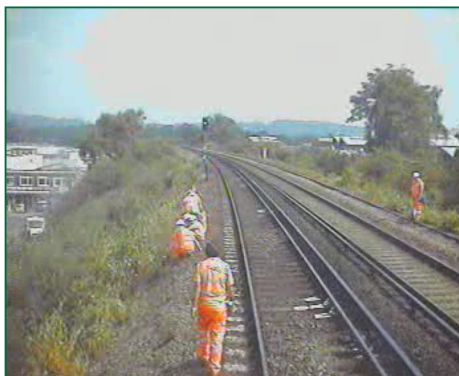
Figure 2: image from the train's forward facing CCTV, immediately before the accident, showing the section supervisor walking along the side of the line, the members of the gang sitting down on the embankment, and the site lookout on the extreme right of the picture
