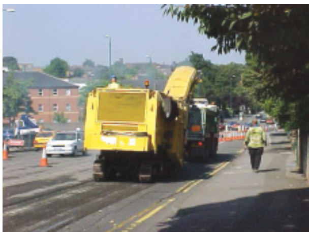
Planing of the carriageway for replacement of the surfacing being carried out under well-controlled traffic management (Source: Nottingham City Council)
