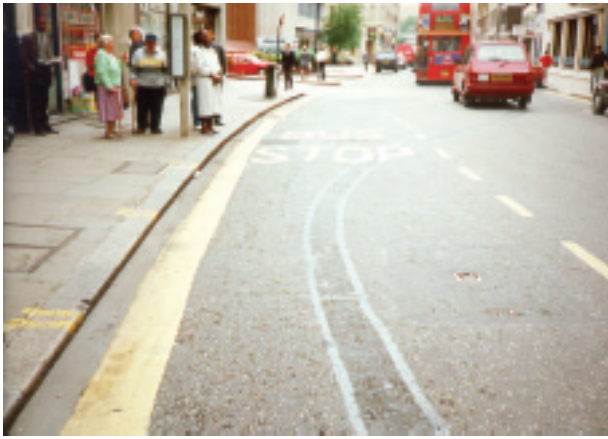
A first-time reinstatement in a busy main street that has been completed to a high standard
