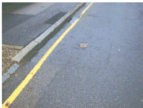
A kerb-line gas industry reinstatement which has been constructed to the surface requirements of the NRSWA (Source: London Borough of Bromley)
