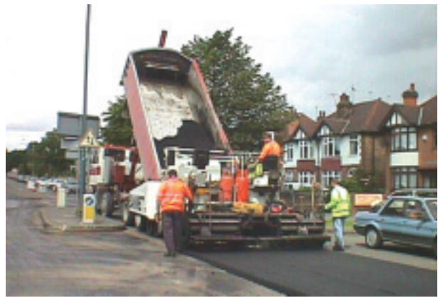
Resurfacing of the carriageway within traffic management control (Source: Cambridgeshire County Council)
