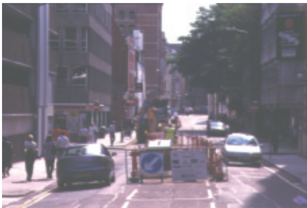
Example of information board and use of two-way traffic for road users (Telia) (Source: THUS Telecommunications)
