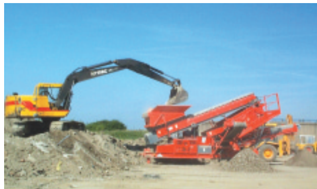
Crushing and grading of material from utility and road excavations for re-use in reinstatements (Source: North West Water)
