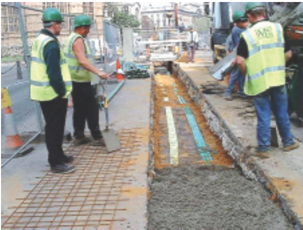
Utility works carried out to the required standards given in the NRSWA Specification (Source: THUS Telecommunications)
