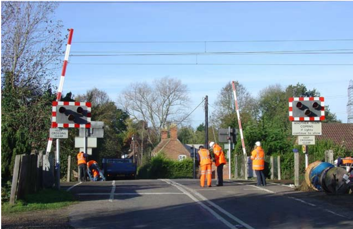
Figure 3: General view of the eastern ( Up side) approach to Swainsthorpe level crossing
