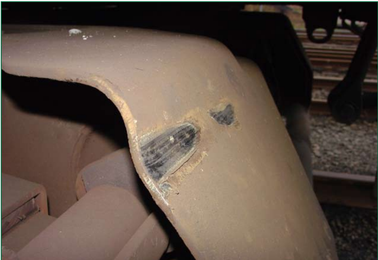
Figure 8: Photograph of deformation of the bogie frame by the wagon structure due to excessive relative movement during the incident
