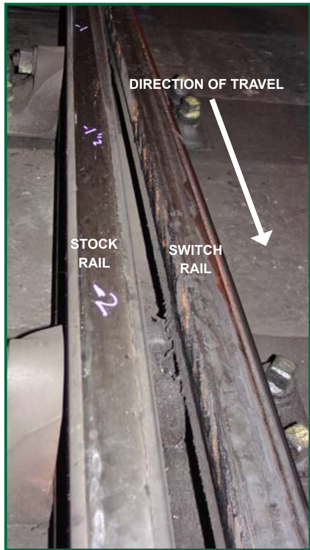
Figure 6: Right-hand switch rail showing wheel marks.
