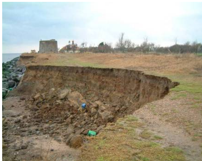
Figure 1.2 Erosion of Environment Agency flood defence embankment, November 2004 (source: Terry Oakes Associates Limited)
