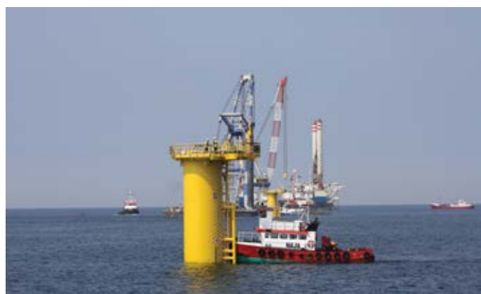
Danish company Blue Water Danbrit UK invested in the Humber in 2011 to provide logistics services for the UK wind industry.
