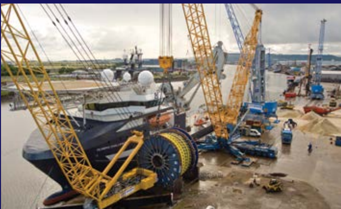
Subsea vessel mobilisation at North Sea Supply Base, AV Dawson Logistics hub and fabrication yard, Middlesbrough
