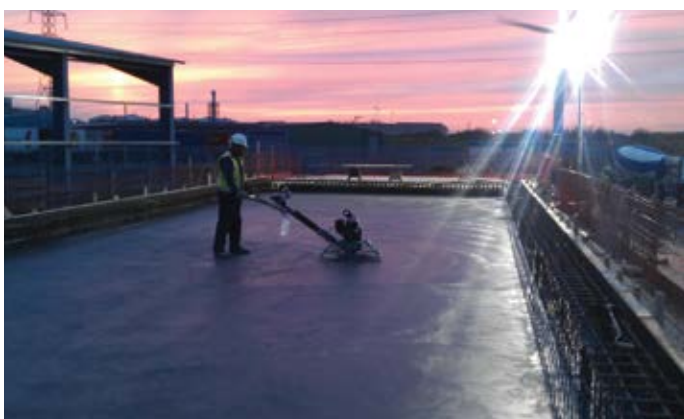
Specialist engineers Spencer Group delivering civil infrastructure works for the onshore substation, to feed electricity generated by E.ON's Humber Gateway Offshore Wind farm into the national grid.
