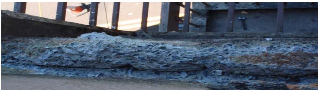
Picture showing bent rebar in wrong area of the concrete
