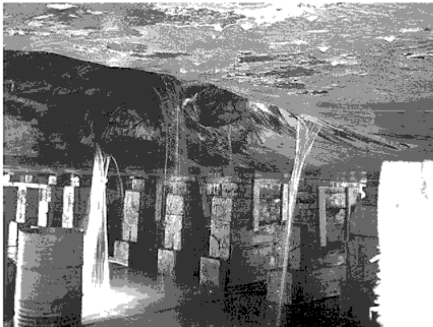
Bottom damage to vessel
