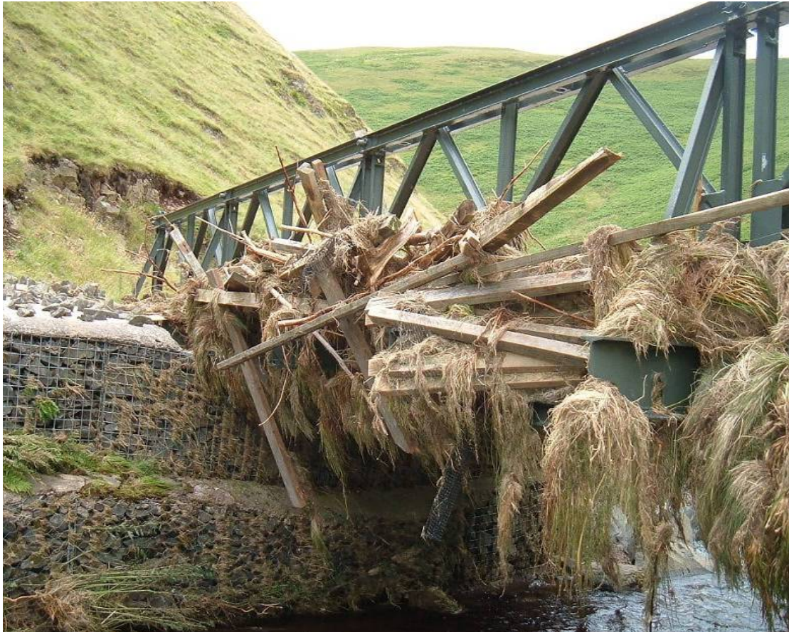
Figure 7 Bridge (in the photo), track and riverside damage by flash flooding at DTE Otterburn caused training disruptions and increased relief costs
