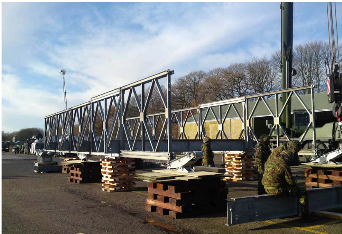
Figure 2 Soldiers from 3 Armoured Engineer Squadron work on the temporary footbridge to span the River Derwent (Cumbria) after severe floods in Nov 09 damaged various bridges across the area leaving communities with no easy access to essential services. The UK CCRA has identified that there would be added burdens on UK emergency services in responding to more frequent flooding, heatwaves and wildfires (Picture: Kevin Hegarty, Crown Copyright/MOD 2009).
