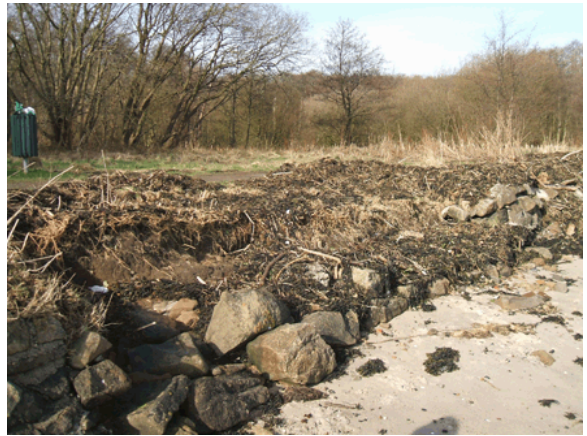
Plate 4: General Damage in Northern Portion of Bay Area
