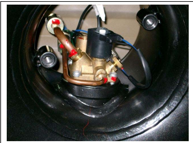
Electric Valve in Under-slung Tank (with cover removed):
