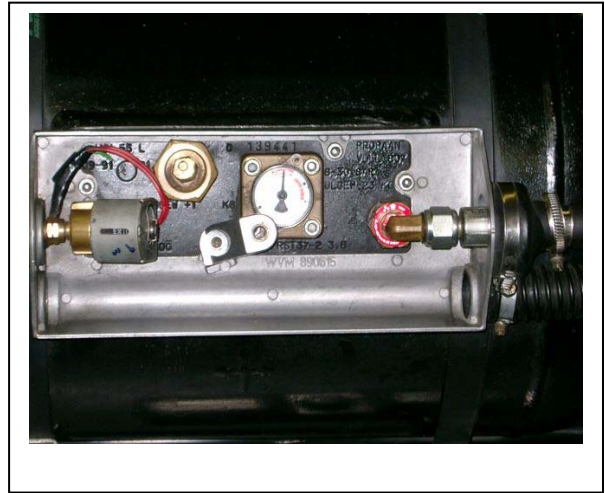
Electric Valve on Cylindrical Tank:
