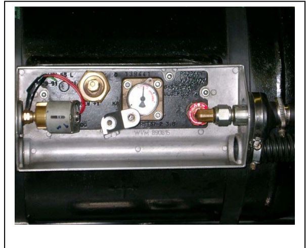
Electric Valve on Cylindrical Tank:
