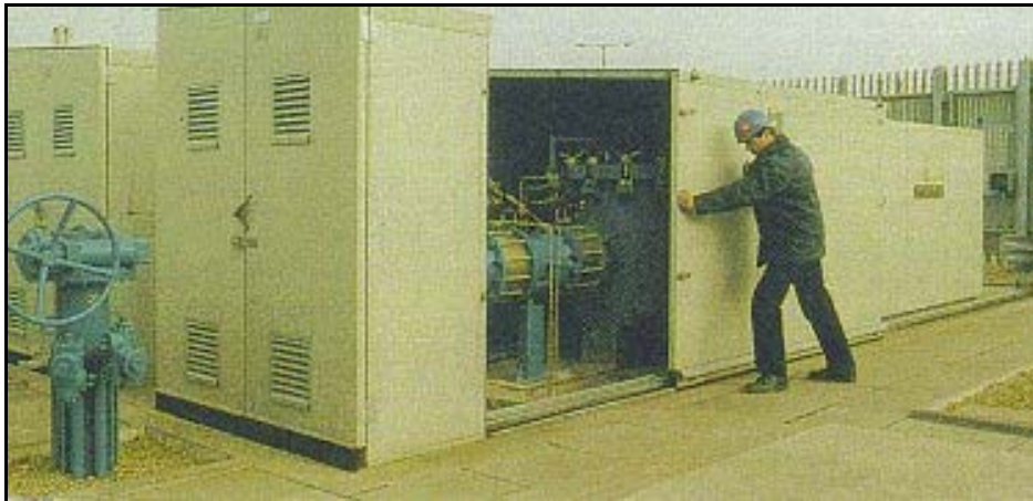
Picture used with the permission of Industrial Acoustics Ltd
