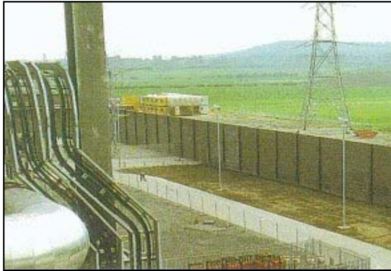
Picture used with the permission of Industrial Acoustics Ltd
