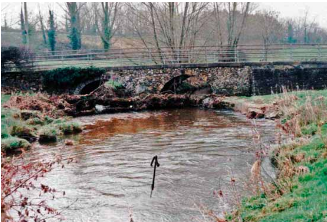
↑ Clapper Lane Bridge: a tree is carried down by flood waters and needs to be removed
