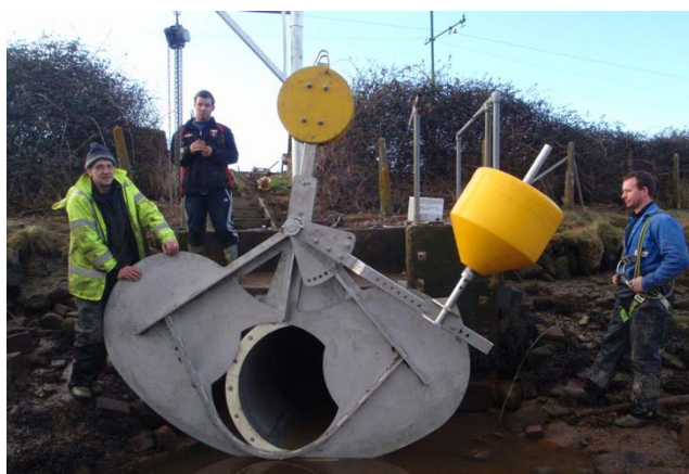
Figure 7: Installation of prototype nearly complete. Note hoist on gantry to assist with assembly.
