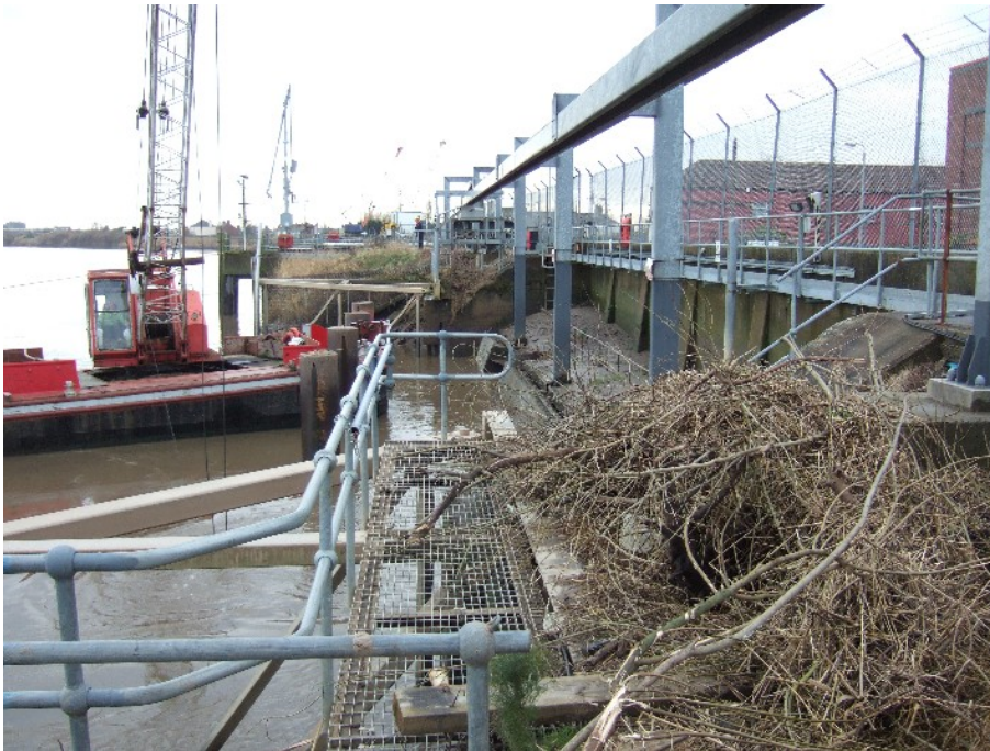
Figure 5-3 CW intake at Keadby, showing overhead gantry rail for screen raking system and accumulated brushwood
