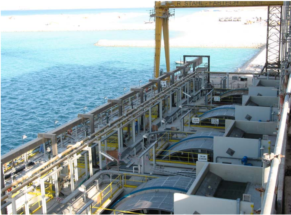
Figure 5-9 Overhead view of typical set of four drum screens at a coastal plant
