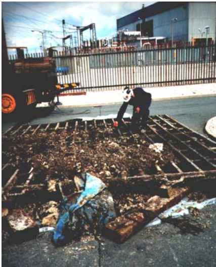
Figure 6-4 Coarse screen blocked by fouling
