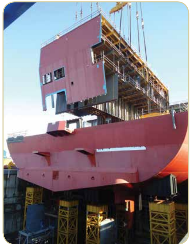
Above: aft flightdeck section installed – one of the final three sections of flight deck (CB05b) was installed on Queen Elizabeth on 10th May
