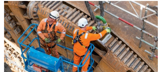
Dorothy completes her second drive under Long Itchington Wood to complete the twin tunnels.
