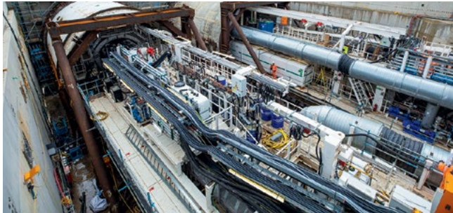
The first London tunnelling machine, Sushila, begins its journey towards the capital, shortly joined by Caroline.
