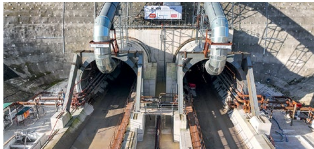
The two Chiltern tunnelling machines, Florence and Cecilia, reach the halfway point of their 10-mile journey.
