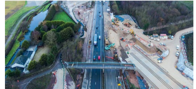
A bridge over the M42 is successfully slid into place, the longest box slide in the world.
