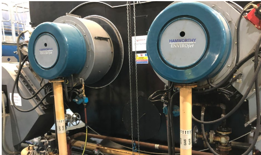
Figure 6 2: Twin Hamworthy burners firing into Danstoker boiler
