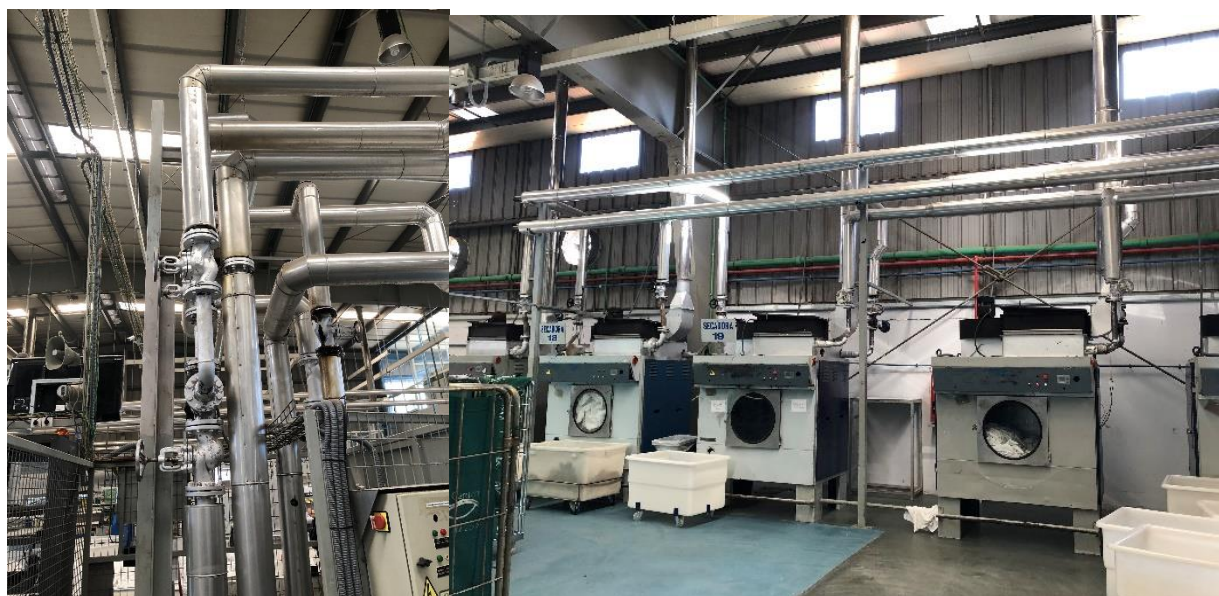
Figure 3: Washer/extractors and a thermal oil piping network. Reviewing the real time data alongside the theoretical energy duty cycles has enabled the peak operating demands of the three model laundries to be calculated.
