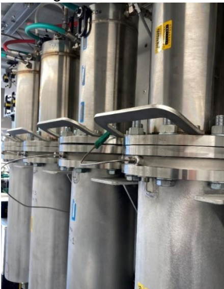
Figure 2: Combined steam generators
