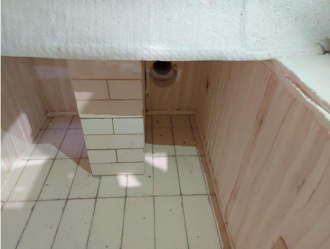
Area a burner. No damage viewed
