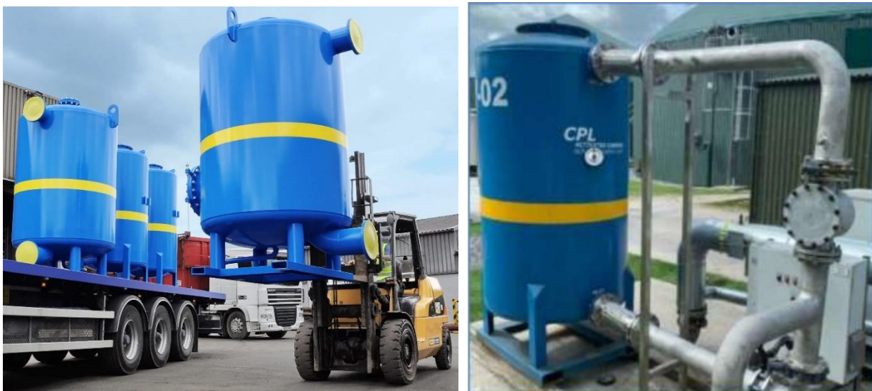
Figure 4 - CPL Gas Purification Units being loaded (left) and in operation (right)
