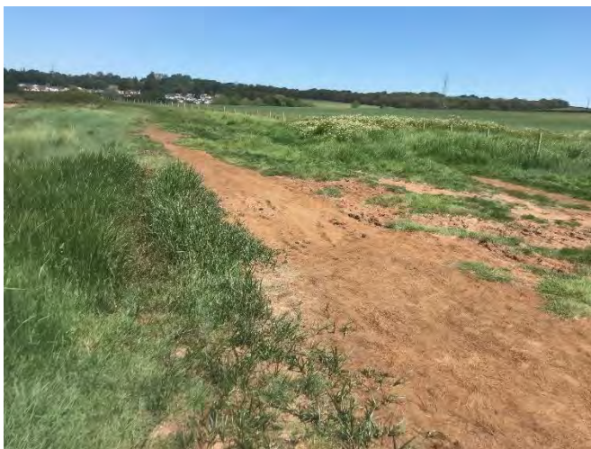
Picture showing muddy pinch point at IOW-10-S060, taken on 9 June 2021. The path is squeezed at this point between the fence and saltmarsh (the patch of darker coloured vegetation on the left of the picture), which needs addressing to make it useable in the winter.
