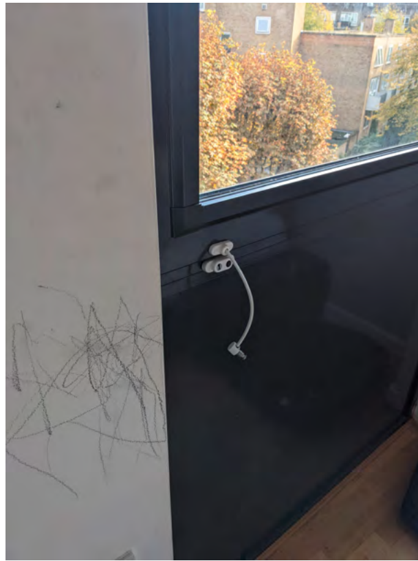
Figure 18: A broken or disconnected window restrictor in an apartment visited by inspectors, which had been used to accommodate families with children
