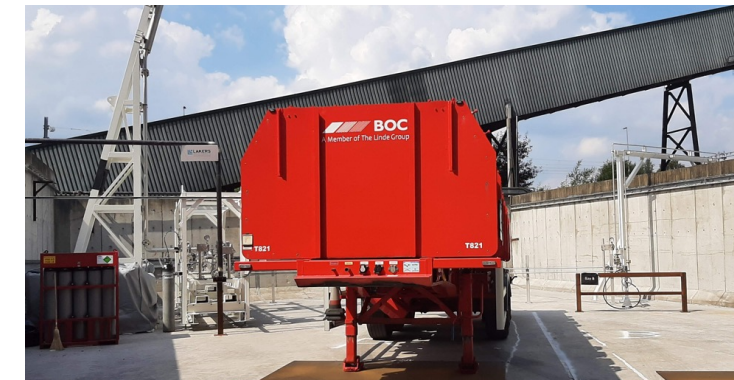
Figure 3.2: Tube Trailer with Primary Pressure Let-down Station
