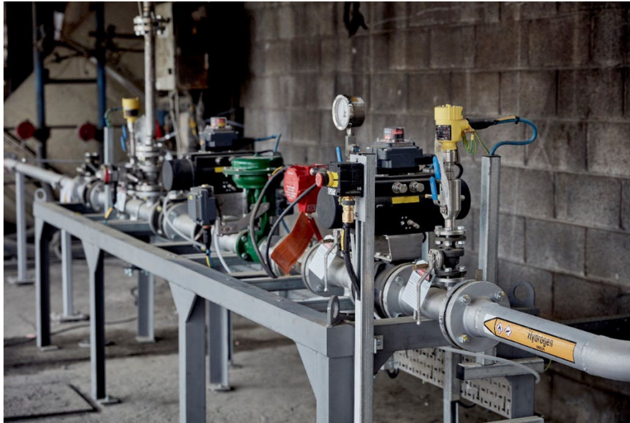
Figure 4.4: Kiln platform hydrogen “valve train”.
