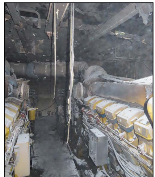
Figure 1: The auxiliary engine room following the fire
