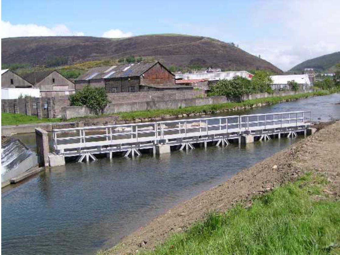
Figure 4.1: Fixed panel screen installed in 2003 on the River Afan, Port Talbot, to prevent salmonid smolts from entering the docks' feeder.
