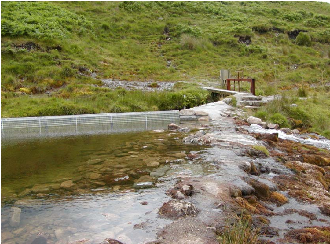
Figure 4.2: Fixed panel screen installed in 2003 on the River Plym, Devon. It protects the entrance to an industrial supply offtake.
