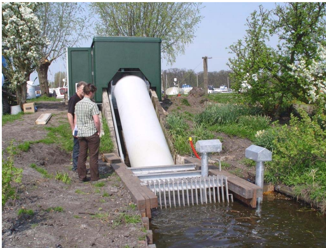
Figure F5.10. Fish Flow Innovations Archimedes screw pump at a pumping station at Zwanburgerpolder, Netherlands. Photograph courtesy of Fish Flow Innovations.
