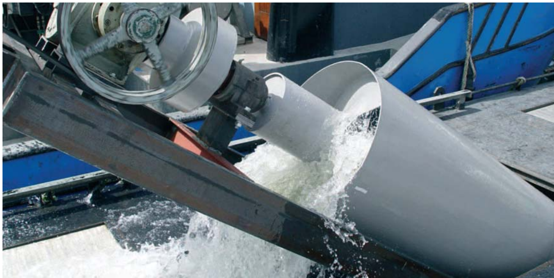
Figure F5.9. Top end of an Archimedes Screw pump with a fixed tube or shroud throughout its length. Photograph courtesy of Fish Flow Innovations.
