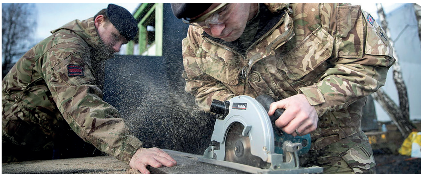
32 Engineers Regiment use specialist carpentry skills to build the first prototype concept Observation Post
