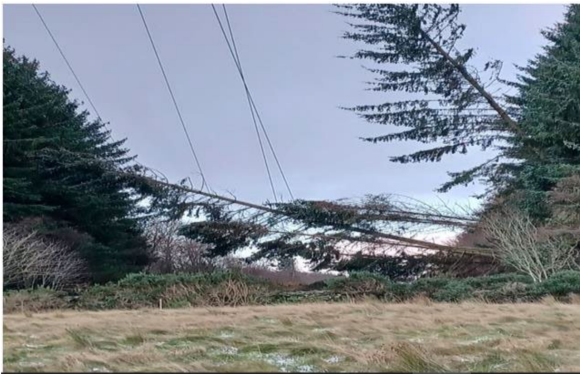
Trees fallen onto lines near a 132kV transmission substation during Storm Arwen
